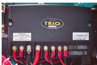
Tank is equipped with water level sensor when is full it will auto stop
