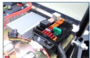
Electric control fuse
